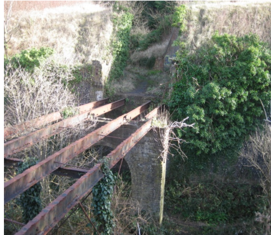
Decaying Bridge near North Entrance
