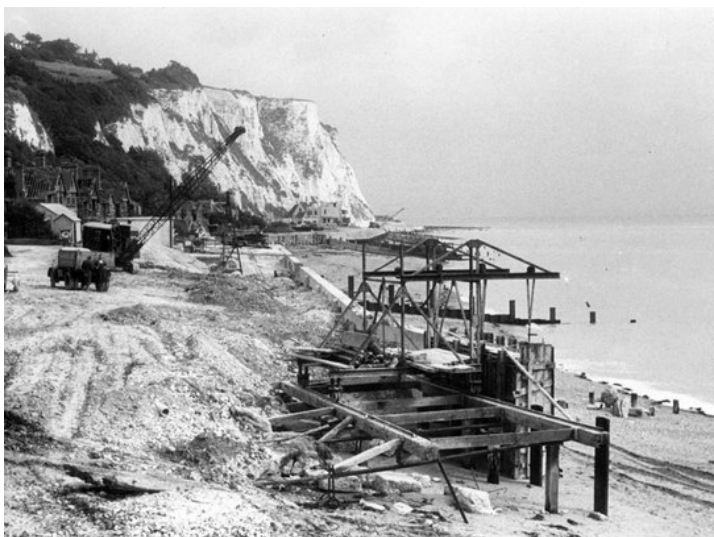
Photograph showing the construction of the new sea wall circa 1951 (Tim Whitaker)
