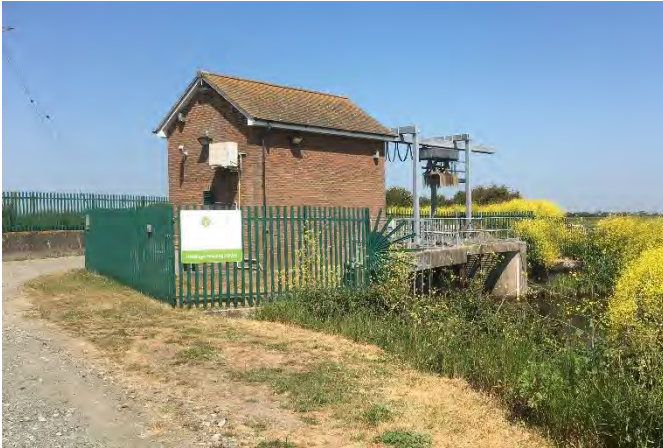
Hacklinge pumping station
