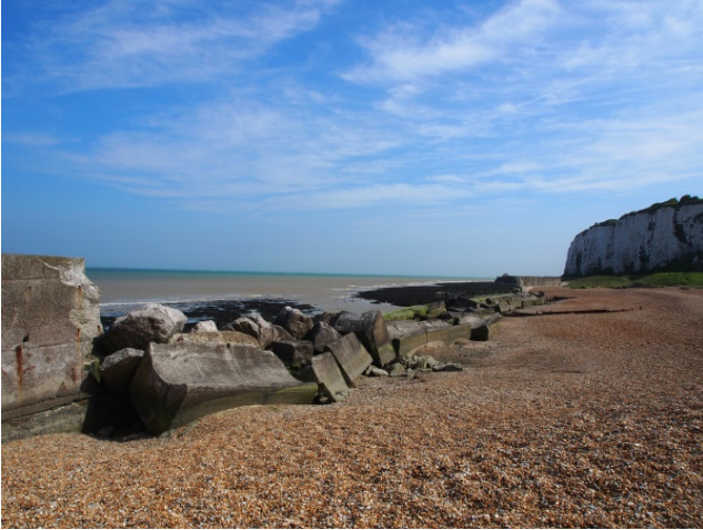
Seawall toppled by storm, Kingsdown
